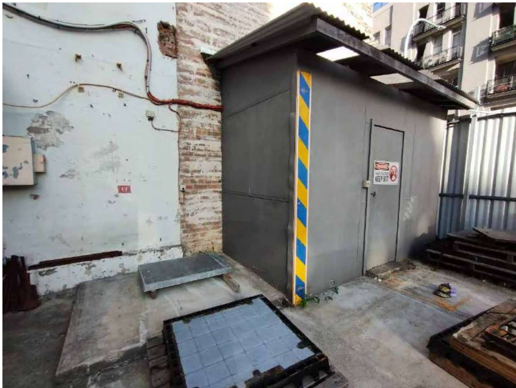
Photo 6: Electrical kiosk with high voltage on an elevated concrete slab located in the north-west corner of the site
